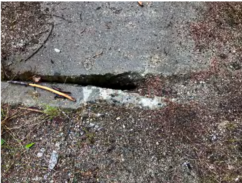
Damage to deck panel and ballast wall
