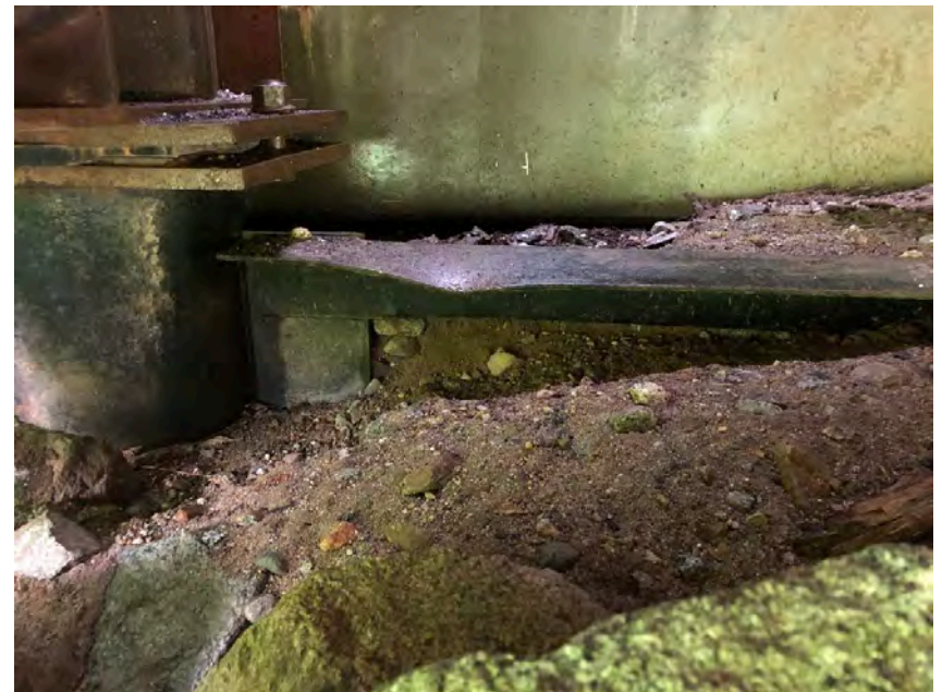
Minor damage to right bank abutment bracing
